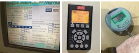
HMI control view illustrating defrost selection and temperature SP.
